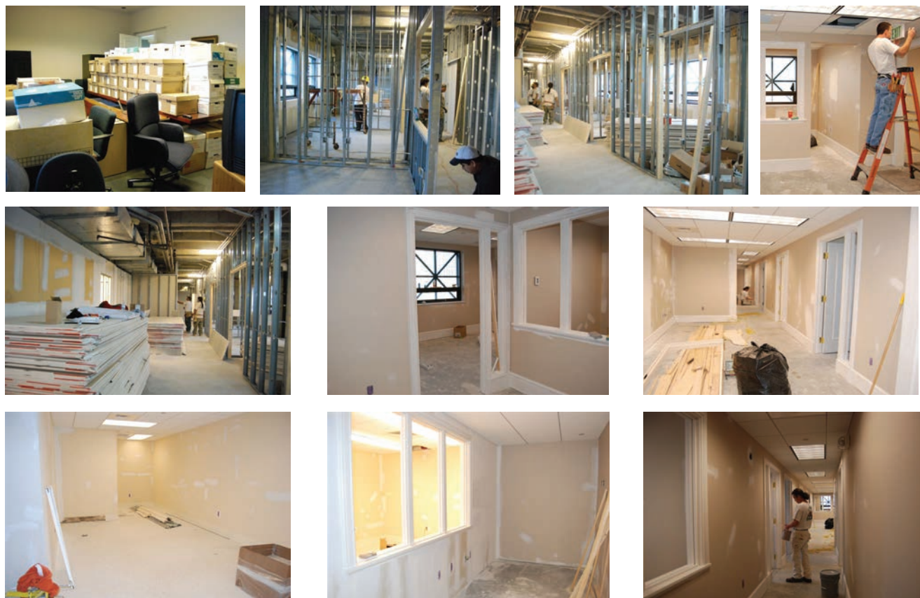
ASB Foundation Assistant Ann Rittenour was designated "clerk of the works" to oversee this project. These photos offer a glimpse at the different phases of construction from framing the office and storage space to wiring the electrical to finishing the walls.
